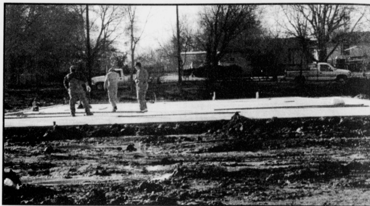
FOUNDATION -Though the weather has not been cooperative, the foundation for the new Talco Post Office has been poured and work continues toward the building. Postal employees hope to be moved into the new location this spring. (Staff Photo Nancy Brown)
