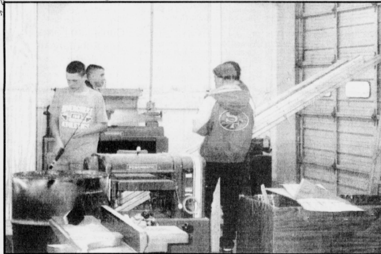
WORKING-on the construction of a storage building in the Rivercrest Ag. Mechanics class are; (left to right) Stephan Cannon, Joey Taylor and Chad Goodwin.
