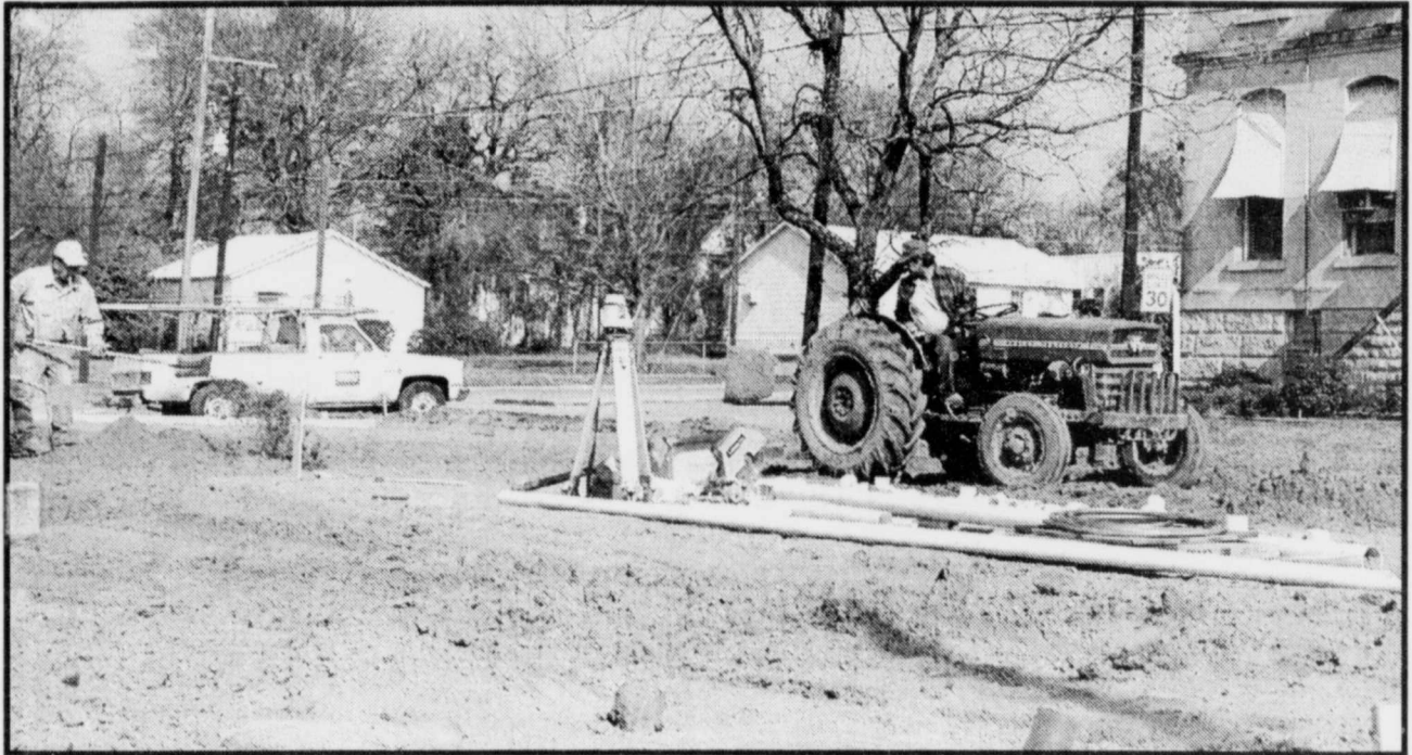
NEW BUILDING-this building near Red River County Jail will be used by company to house a business which will utilize inmates from the jail. (Staff Photo by Thomas Nichols)
