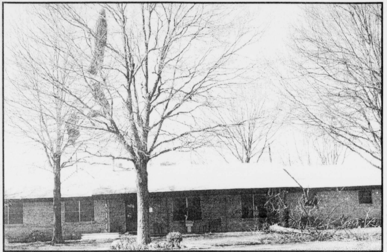
A STORM-rolled through the Talco area Saturday night around 9:00 p.m. and did its share of damage. The home of Mrs. Alex Waddell had the carport destroyed, rain gutters and vent turbines torn off and a tree laid down. Damage was also done to the home of Terry and Patty Jones across the street from Mrs. Waddell and the carport on the Wake Wood home was also lifted and deposited behind Mrs. Waddell's home. No one was injured in the destruction. (Staff Photo Nancy Brown)
