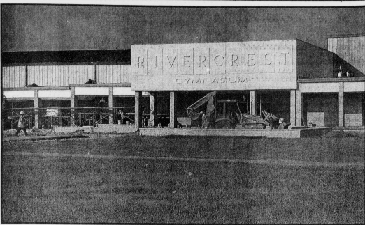
REBEL GYM will be ready by the time basketball season arrives according to contractors. The new structure will be a source of pride for coaches, students and members of the communities. (Staff Photo Nancy Brown)
