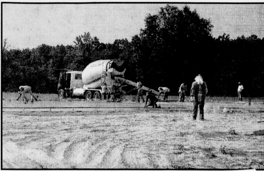
NEW BUS BARN AND ISS/AEP CLASS ROOM -Workmen were busy Tuesday pouring concrete for the new bus barn and ISS/AEP class room. The new facility will be a great improvement for those students who are unfortunate enough to make use of them and the new bus barn will be a very nice move for Transportation Director, Ricky Kennedy and staff. (Staff Photo Nancy Brown)
