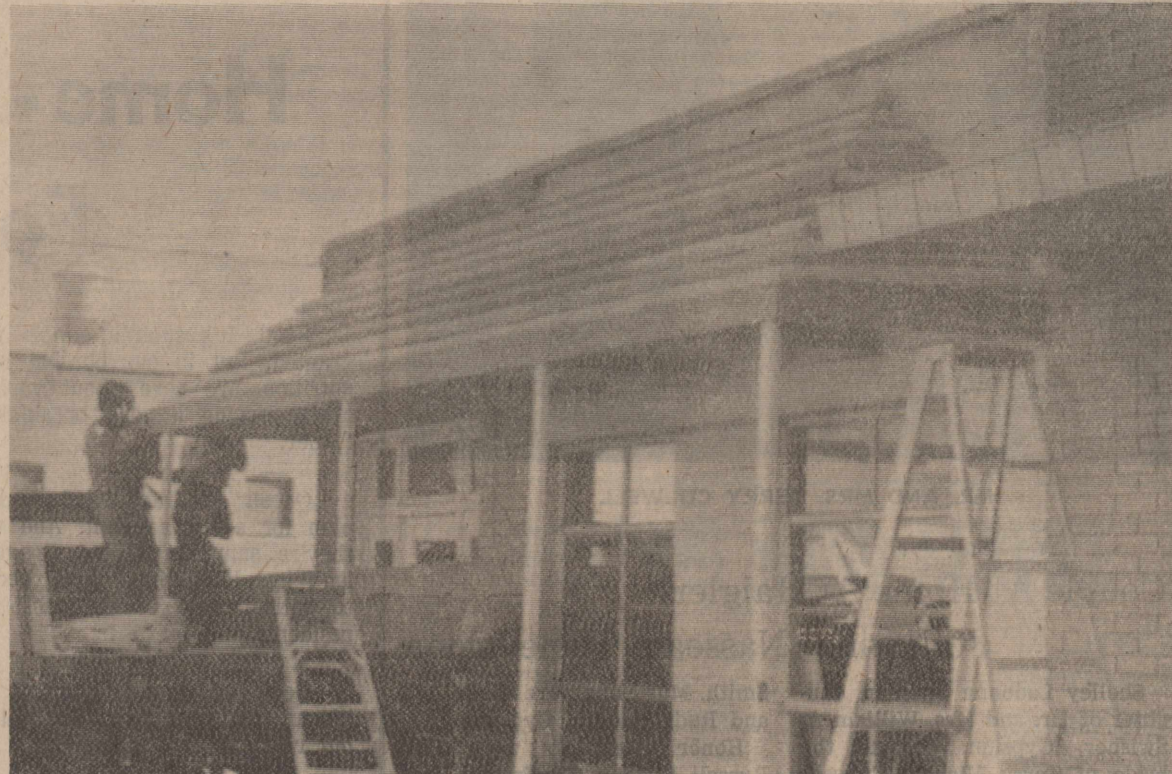
Work is in full swing at the old post office building which was purchased recently by Riley and Sandy Harris. A new front and other remodeling are being done for the Harrises by Fogerson Lumber & Supply. A new business will be housed here when the construction has been finished. (Briscoe County News Photo)
