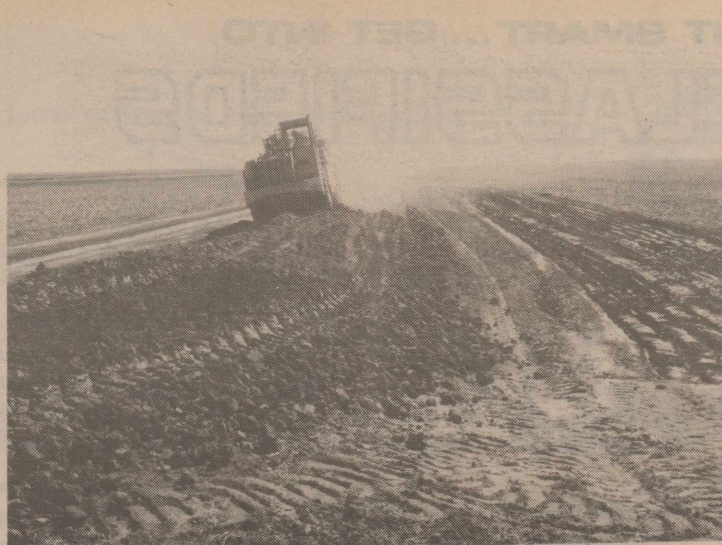
Terraces aid in stopping these erosive gullies.
