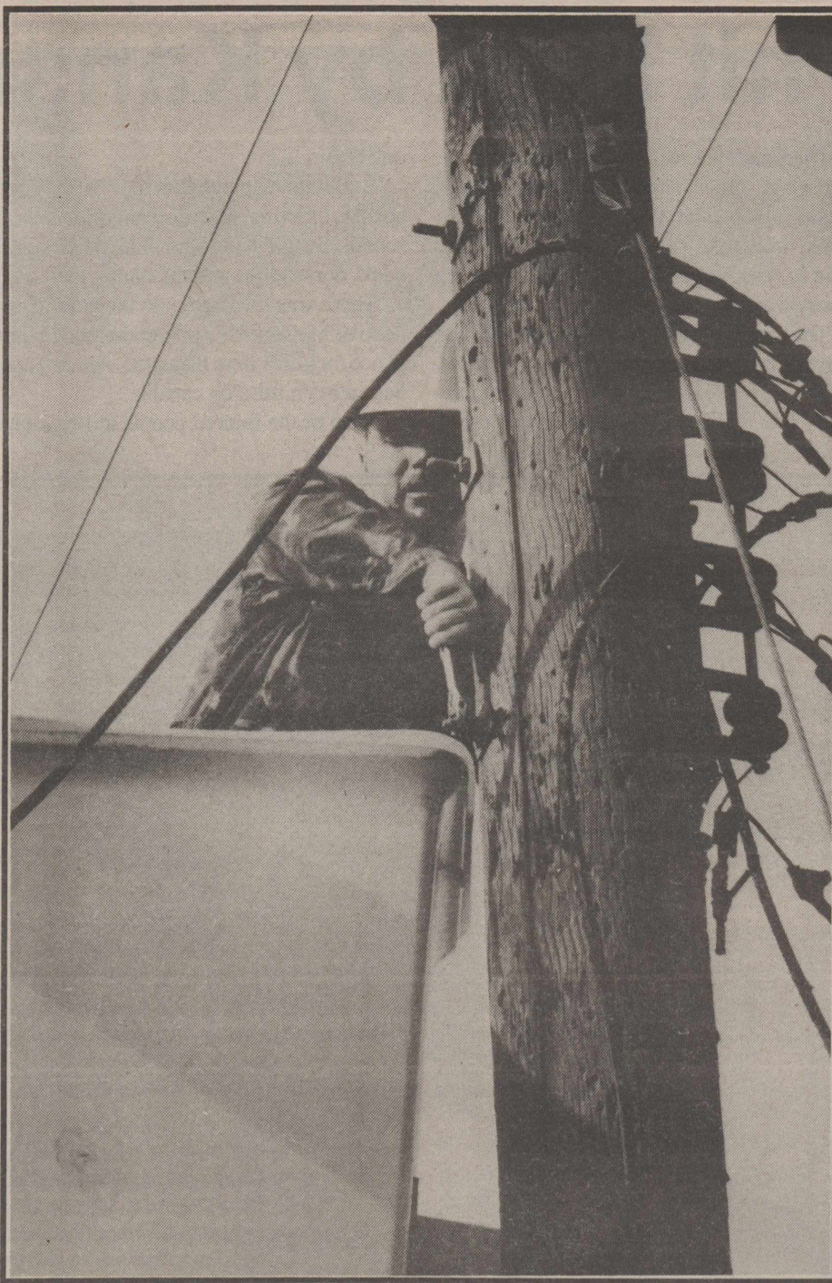
(Sgt. Greg Spraggins) Sgt. Tim Givens, 64th Civil Engineering Squadron, works on one of the base's power poles.
