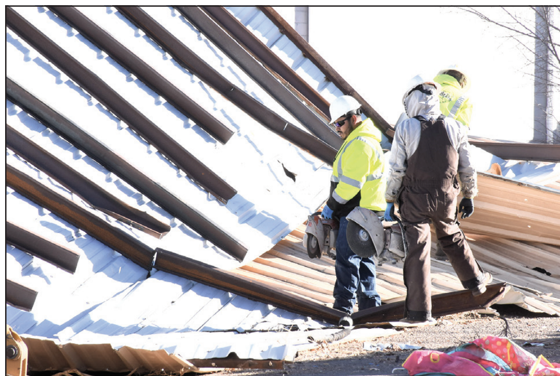
Wind Damage in Friona — Around 1:15 p.m. last Sunday the roof was torn off the American Legion building at Euclid & 6th Street by a windstorm
