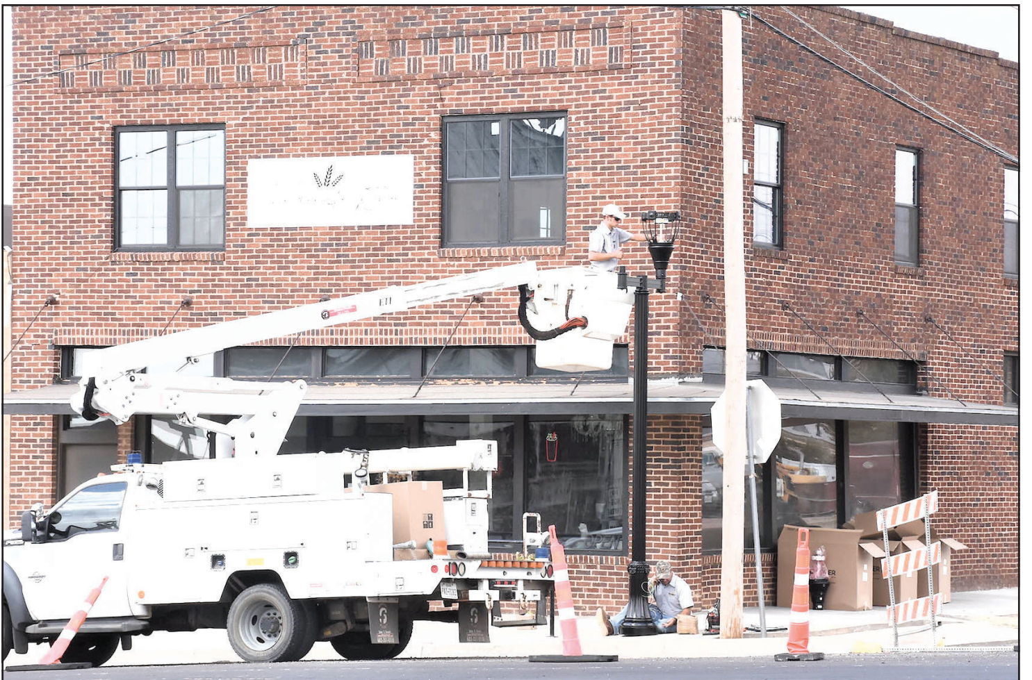
Charles Cooper (bucket above) and Stephen Campbell (sidewalk below) of Campbell Electric are shown installing a streetlight at the corner of 5th and Main in front of The Farmwife Kitchen restaurant. The lights are part of the Downtown Revitalization Project partially funded with grant money. The number of streetlights installed was scaled back from the original plan due to the pandemic and high inflation that drove prices up.
