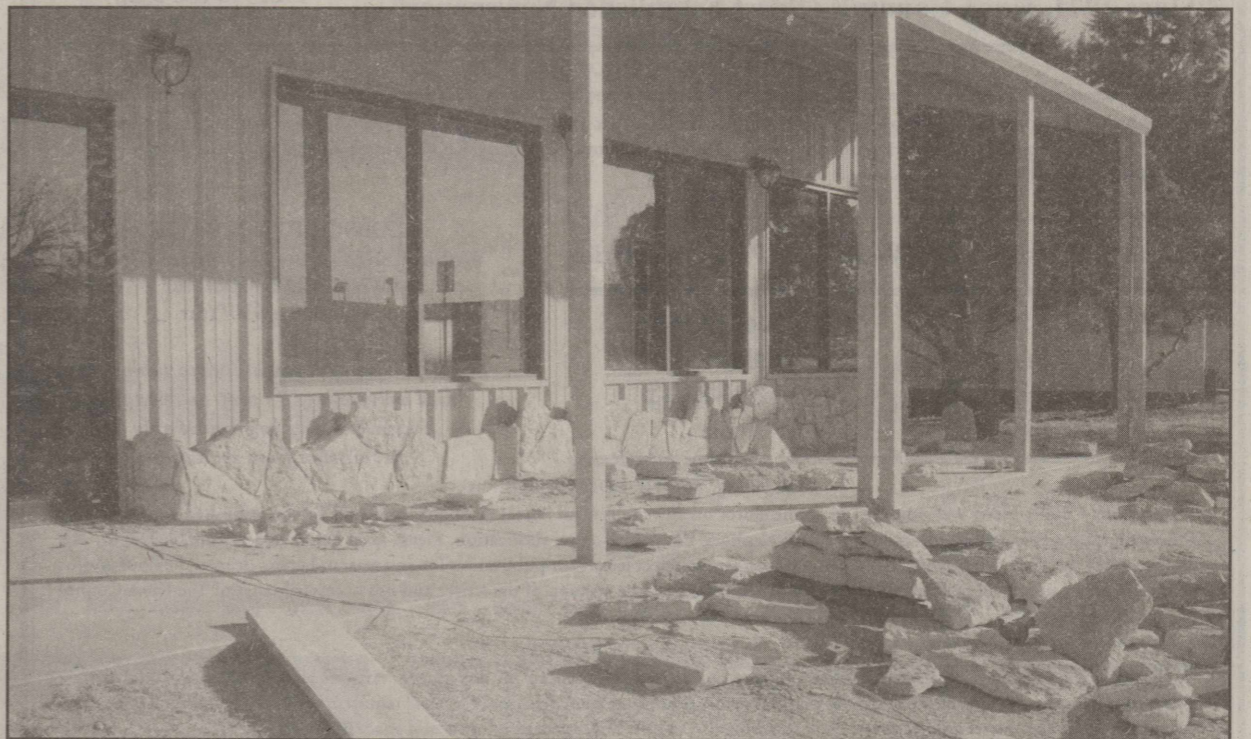
The rock exterior is being placed on the Knox County Museum exterior. Dale Huffman and Kevin Urbanzyck of Munday started work last week.
