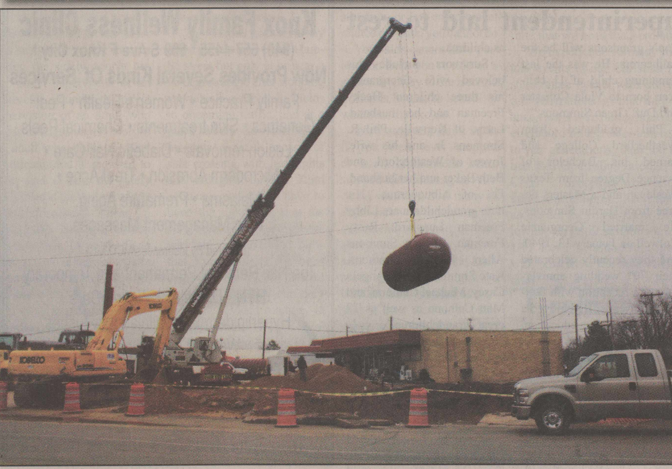
A huge tank is lifted into the hole. This tank will become one of the reservoirs where diesel will be stored until it is dispensed at the pump to paying customers. (Photo by Tamara Smart)
