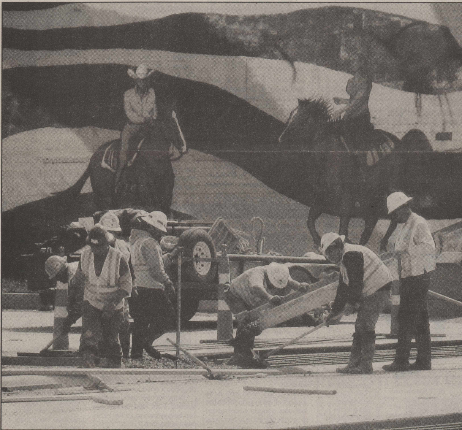
Road construction crews smooth out part of the concrete they applied to the roadway on Central Avenue on Tuesday morning. Construction crews have paved a portion of the road, and are expecting to complete the first half of the downtown paving project within the next few weeks.
