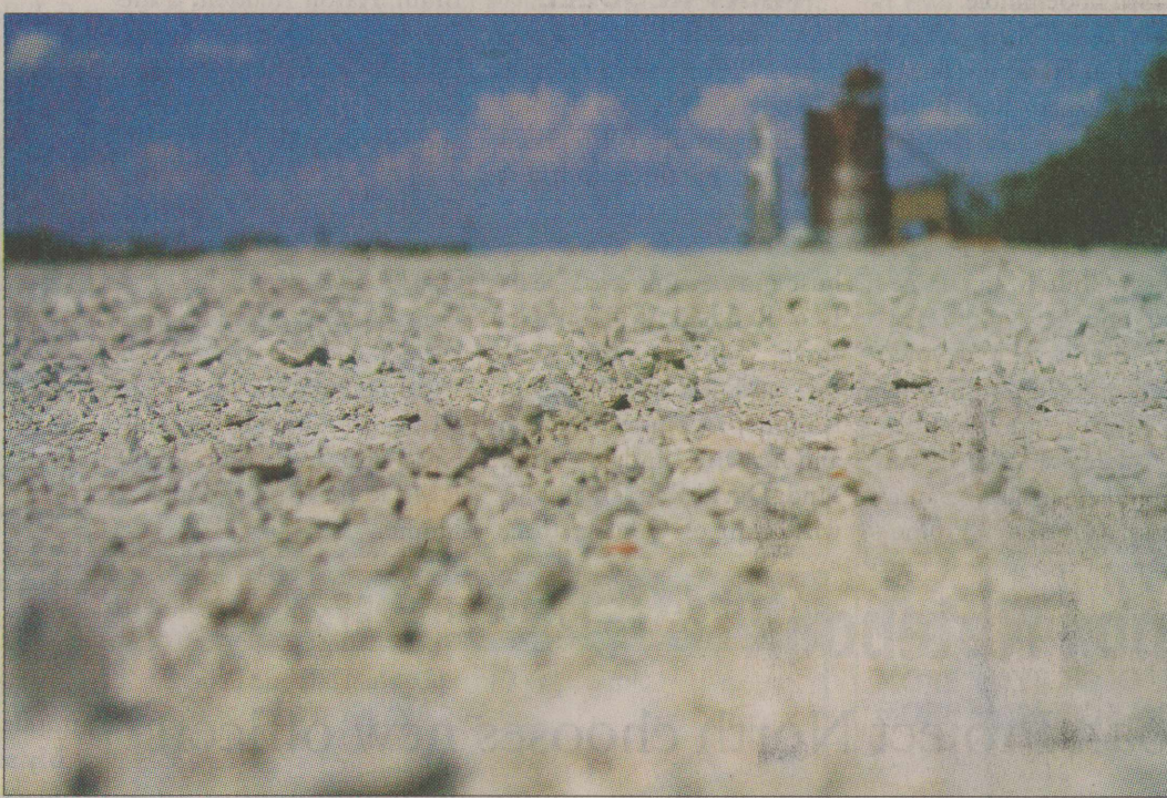
Wayne Hodgkin/The Knox County News-Courier Fresh gravel was recently poured onto what will become the northbound lanes of U.S. 277 through the Bomarton community. The new four-lane, divided highway is being built in several phases between Knox and Wichita counties. The grain silos shown in the background will be razed to make way for the expanded highway.
