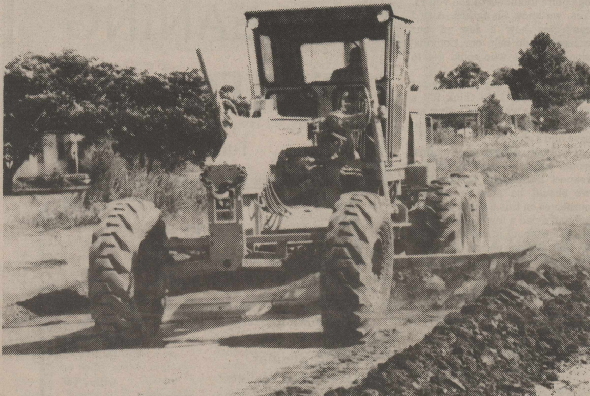
Grover Thomas is shown preparing the roadbed for caliche being put on Stalbird Street. The city is repairing some 13 blocks, making them into all-weather streets.
