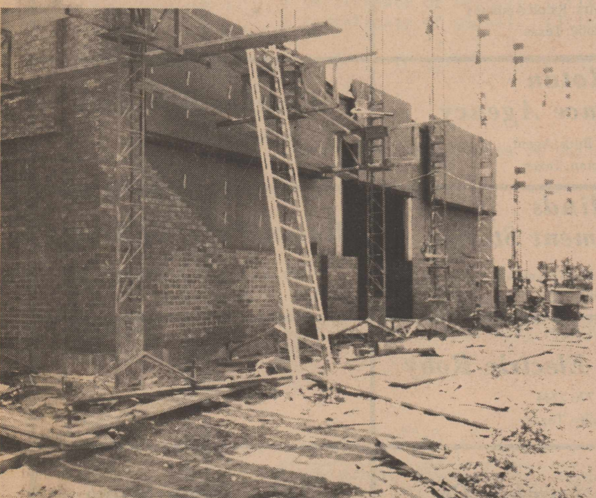
NORTH WING: Brickwork is about 50 percent completed on the north wing and workers are currently installing domestic water lines and constructing interior panels.
