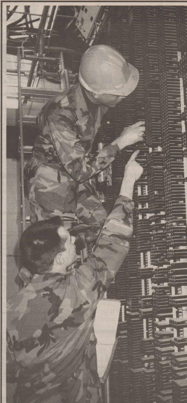
SSgt. James Jewell A1C Charles Bryant, bottom, and SrA. William Stock Jr. perform jumper circuit verification prior to project implementation on the central office distribution frame in Bldg. 20
