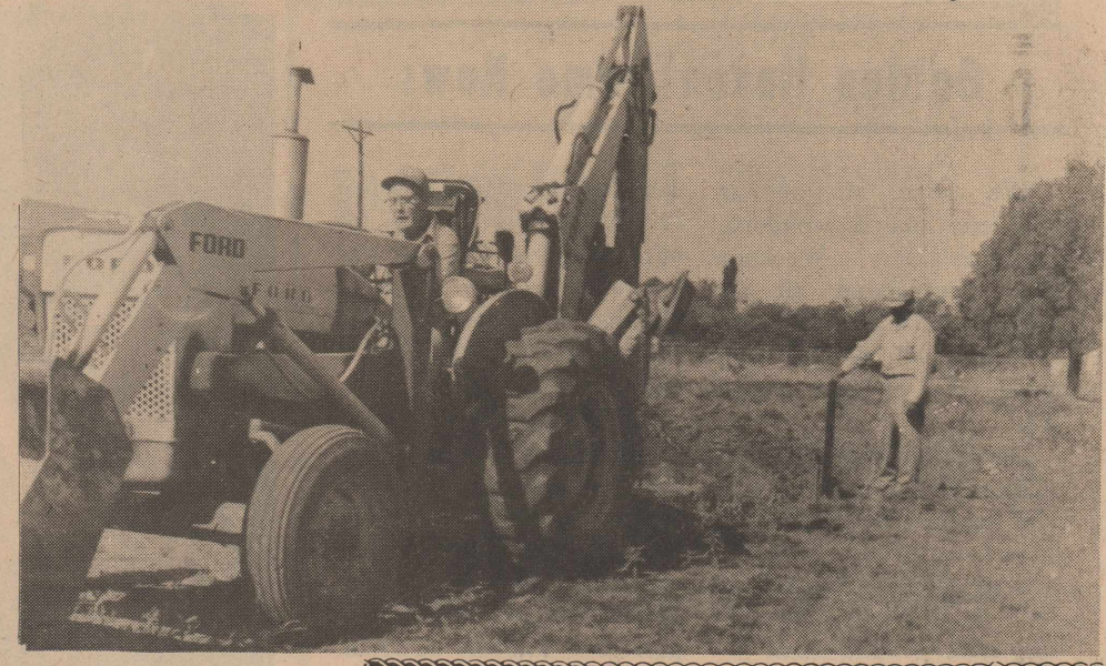
INSTALLING WATER LINE: Zed Randolph, operating backhoe, completed installing a water line to the new softball field earlier this week. Approximately 60 girls from throughout the country are taking part in the Fisher County Softball program.
