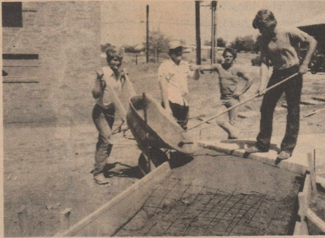
NEW SIDEWALK: Members of the Rotan FFA department constructed a sidewalk from the north end of the school building to the auditorium this week. The project, under the direction of FFA instructor Ronnie Teichelman, is part of a class on cement work. Identified, left to right, Todd Goodwin, Mark Yates, Mark Henderson, and David Posey.
