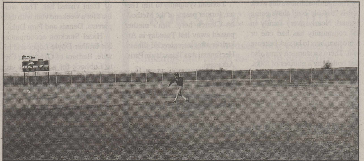
BUILDING A BASEBALL FIELD FROM SCRATCH is no easy task, and work continues at a fast pace to get the new field at Knox City High School's athletic complex ready for the first home game scheduled for Tuesday, March 2. The outfield fence and backstop are finished, the scoreboard has been installed, and the dugouts are nearing completion. The announcer's booth, bleachers, and finishing out the base lines and pitcher's mound are ongoing projects. This first season, Knox City will not host any night games, as the field has no lighting system.
