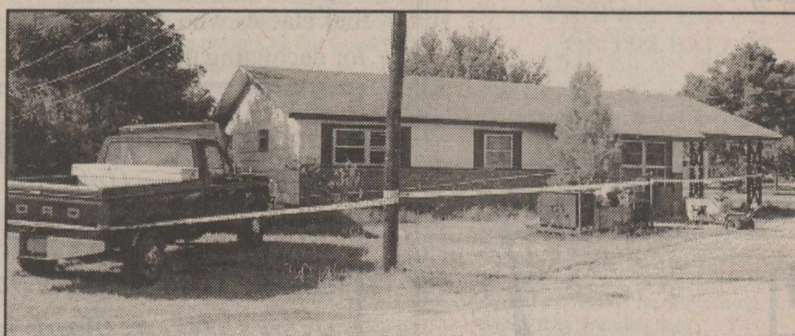
THE CLARK RESIDENCE after the fire, marked by yellow crime scene tape. Local officials are awaiting an investigator from the State Fire Marshal's office to conduct an investigation.
