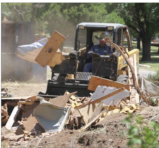
City sanitation director Joe Neal Shadle maneuvers a skid loader during the demolition of a old house on Sully Street last Tuesday afternoon.
