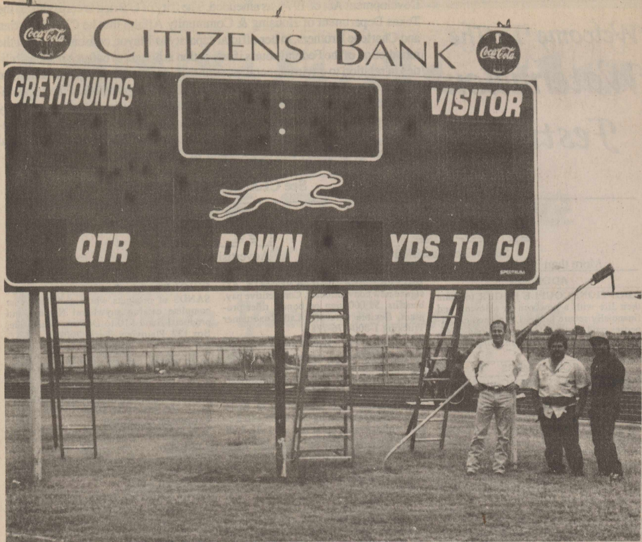
PROUDLY STANDING BEFORE THE NEW SCOREBOARD AT GREYHOUND STADIUM , Citizens Bank President Greg Clonts is shown here with two workmen from Spectrum Scoreboards in Houston who were in Knox City last Wednesday to install the new scoreboard. Both Citizens Bank and Coca-Cola made the new scoreboard possible, replacing a scoreboard that was manufactured back in the 60's. Featuring a new yards to go display for football games, this new scoreboard can also be used as a timer for track and field events with the home time being the minutes and the visitor time being the seconds. (NEWS Photo)
