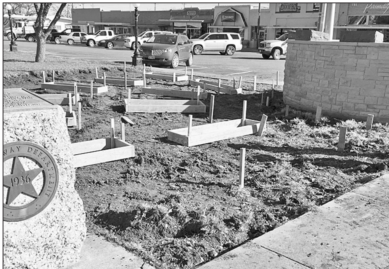
WORK BEGINS —The work has begun for the Veterans Memorial in Haskell. Dirt work and layout of the construction started last week. The memorial will be on the southwest corner of the square and will incorporate the existing memorial and flag pole.
