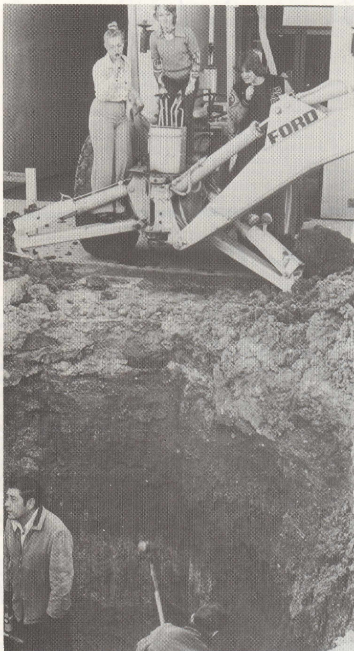
'WE DIG WTC!' — Journalism staffers (L to R) Paula Cornoyer, Jill Groff and Tracy Moore look on as maintenance crew repairs broken water lines between the LRC and Student Center.
