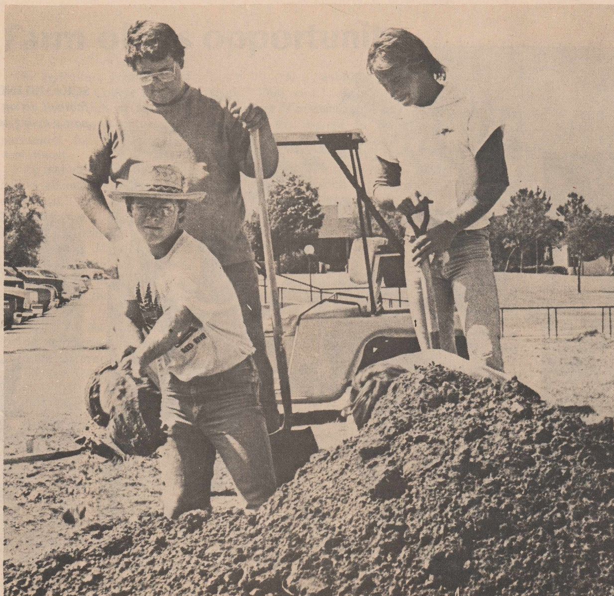
WATER SYSTEM -Tapping into the main waterline in order to install a new sprinkler system are Tim Blanchard of Gatesville, Paul Joy of Abilene, and Robert Bryan of Tulia. -Jerry Snelling photo
