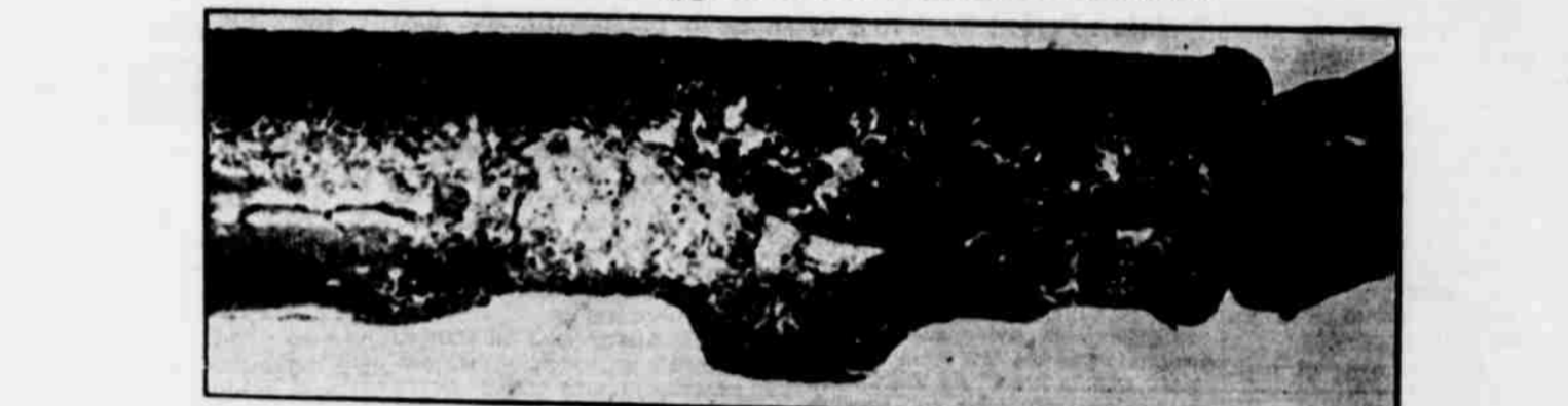
Above: Wire with insulation blistered. Such heating causes energy losses of as much as 25 per cent of light bulb or electric appliance efficiency. Below: A new section of proper-sized wire. These are actual photographs of the wire removed and the wire used in enlarging the circuit in a West Texas bank when it was re-wired to meet the demands of additional lighting and appliances put in use since the structure was built.
