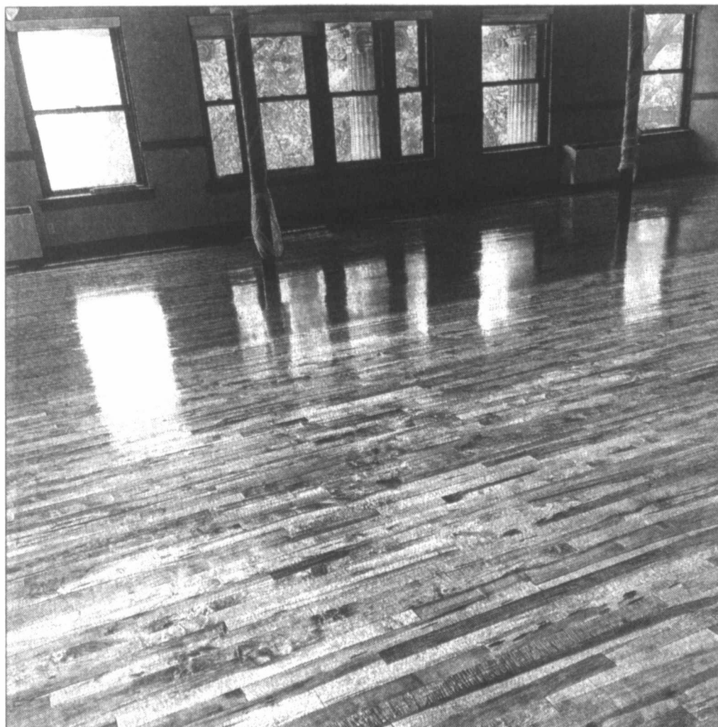
New floor ... The new maple wood floor has been laid and finished inside the District Courtroom on the second floor of the Lynn County Courthouse. The original flooring was ruined when a major flooding incident occurred at the courthouse in May 2021, and the courtroom has been unusable since then. With the new floors laid, the chairs and other furnishings will be installed, and the courtroom will again be open for business soon. During the interim, district court has been held at the Tahoka Housing Authority center. (LCN PHOTO by Juanell Jones)
