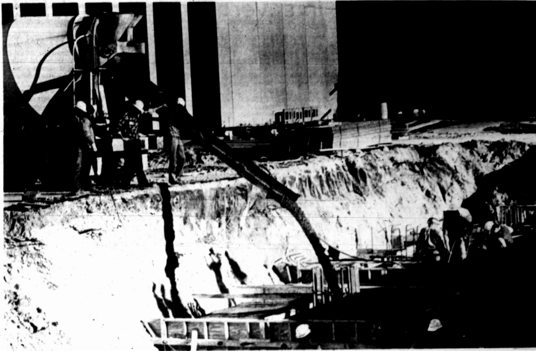
The first 279 cubic yards of concrete were poured Thursday at Midland National Bank's second tower, forming three of the four "footings" that support the building. By the time the 14-story building is completed in December, 17,000 cubic yards of concrete will be used to help construct the office building and adjacent six-level, 780-parking space garage. (Staff Photo)
