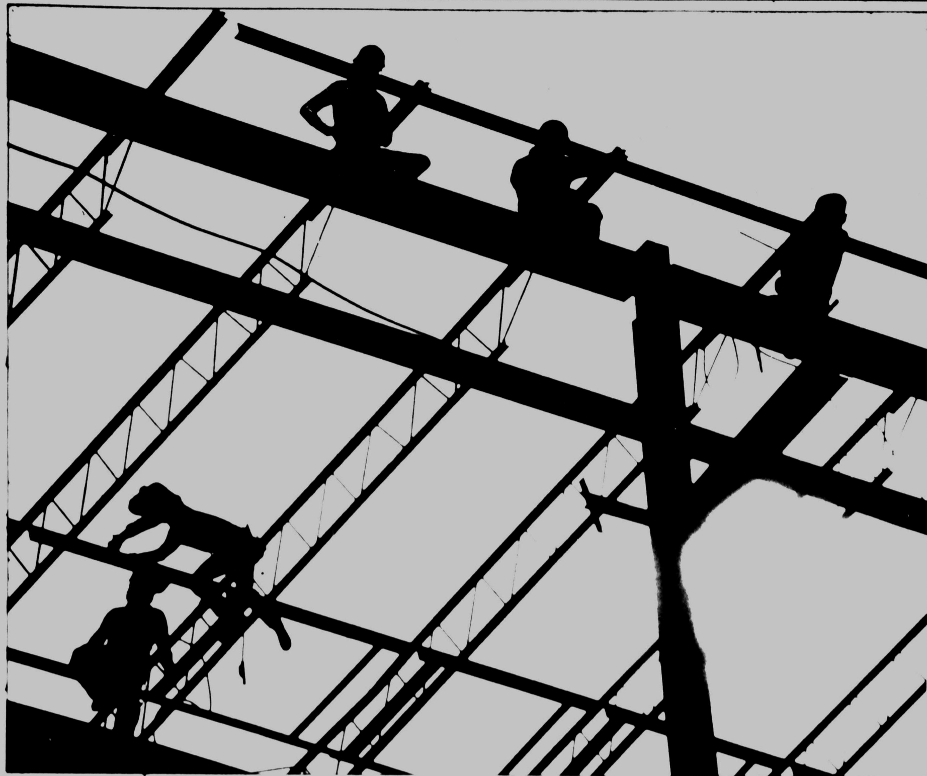
A warm January sun silhouettes welders atop the Paragon building near downtown Midland Wednesday. The Paragon, a 10-story, $18 million building located at Marientfeld Street and Louisiana Avenue, is one of several major office complexes now under construction in Midland. (Staff Photo by Paul Gilbert)
