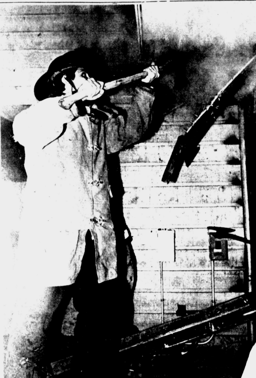
Chopping away part of the burning roof is a city fireman, who was one of firefighters called to a fire at the Silverado Apartments, 2613 N. Midland Dr., about 9:30 p.m. Thursday. The blaze did heavy damage to the walls, ceiling, and floors of two apartments in the complex. A plumber's torch was believed to have caused the fire, which took more than an hour to extinguish. (Staff Photo by Paul Gilbert)
