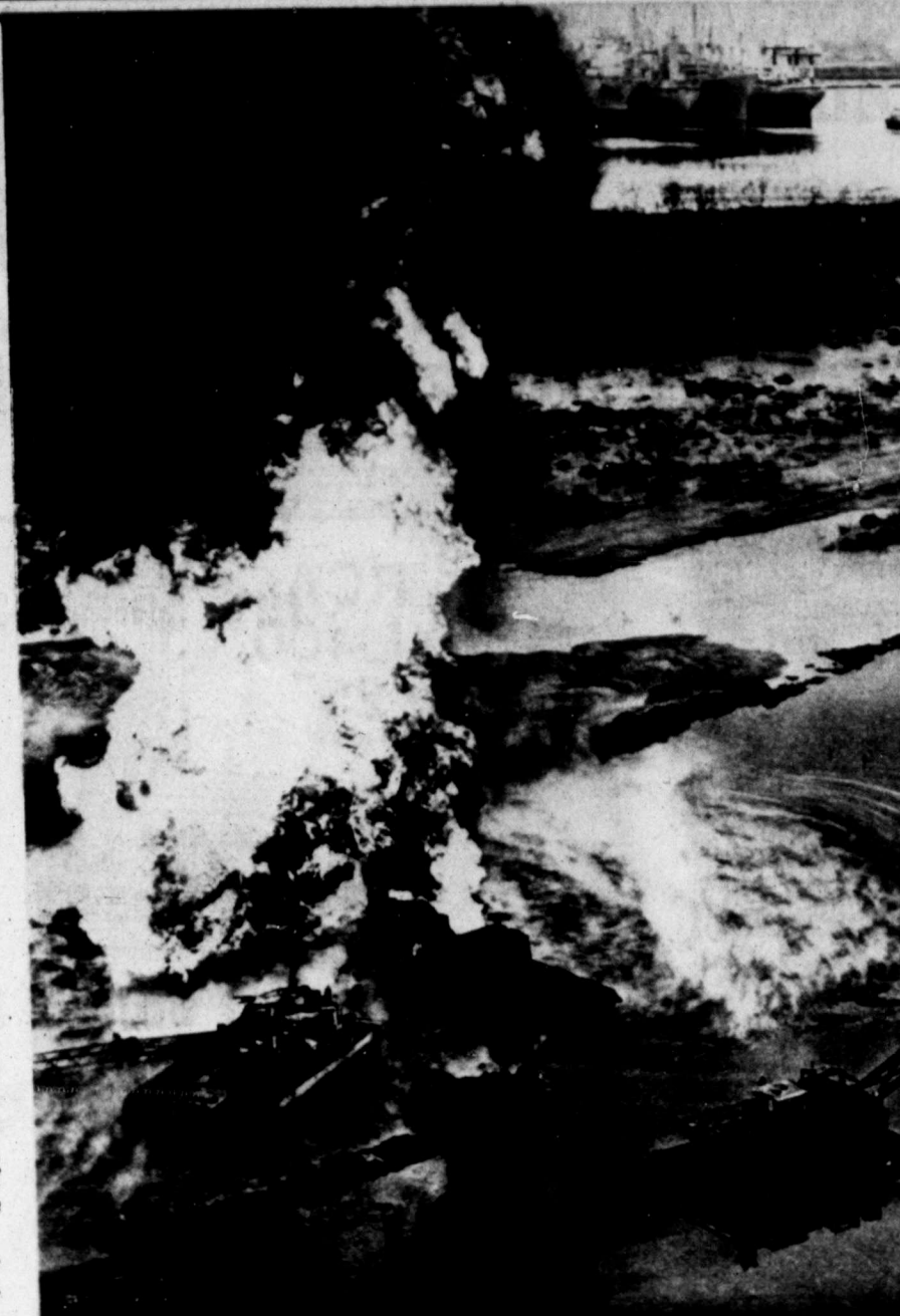
A pipeline carrying ethylene burns in a marsh near the Neches River, Beaumont, after it exploded during construction of parallel line. Three persons were hospitalized after evacuation by boat and helicopter. Pipeline laying equipment is in the foreground and part of a fleet of mothballed World War II ships is seen at upper right. (AP Laserphoto)
