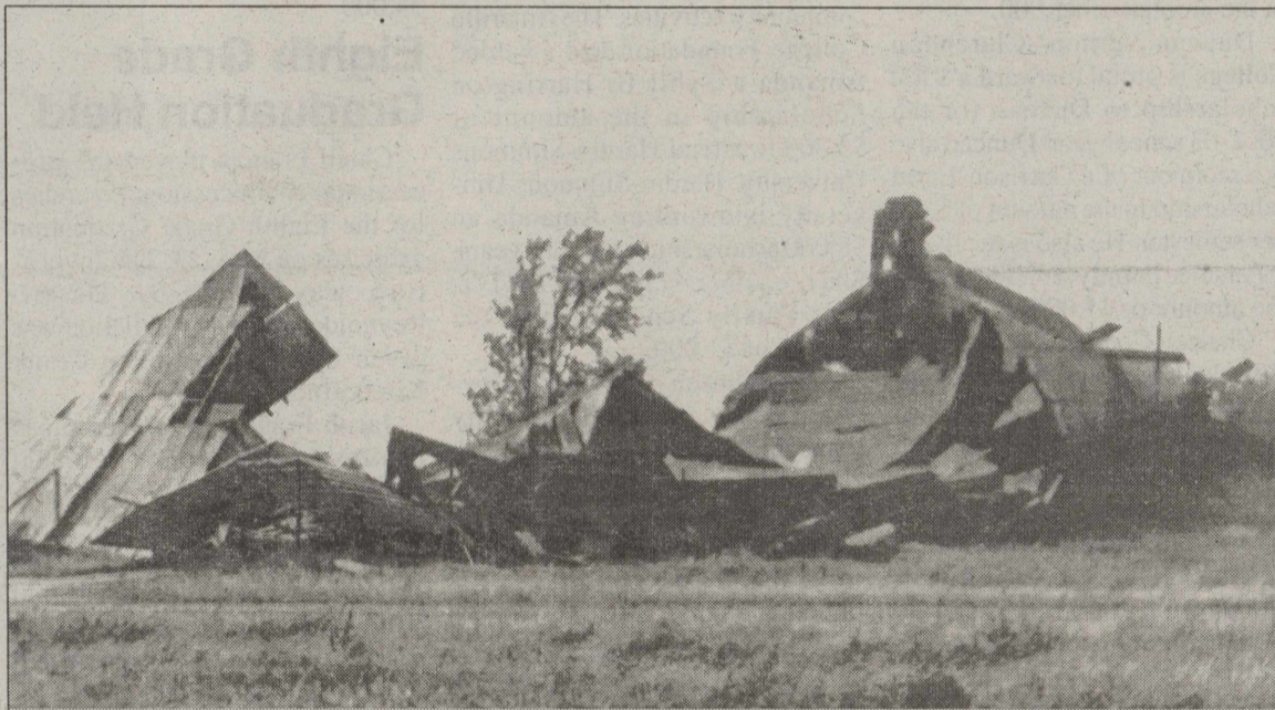
Wind damage was done at the old Harvest Queen Elevator in the northeast part of Silverton Sunday afternoon. Briscoe County News Photo
