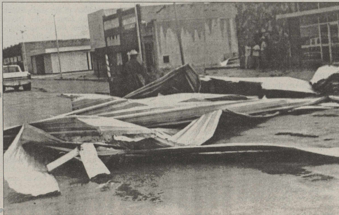
Sheet metal that blew off the roof of Rhoderick Irrigation littered the street of downtown Silverton after a windstorm that hit Silverton Sunday afternoon. Briscoe County News Photo
