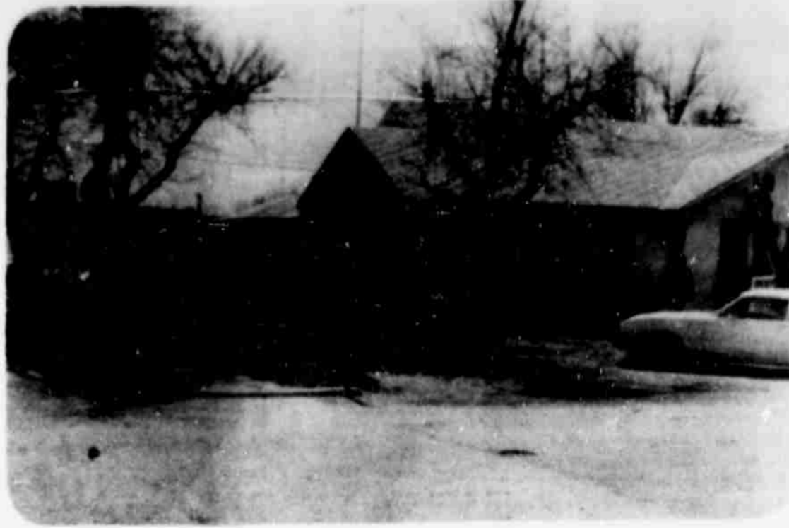
THE YOUTH OF FIRST BAPTIST CHURCH took advantage of an Easter vacation to do repairs and paint the House of Life, which is located across the street south of the Church. (Staff Photo By Don Comedy)
