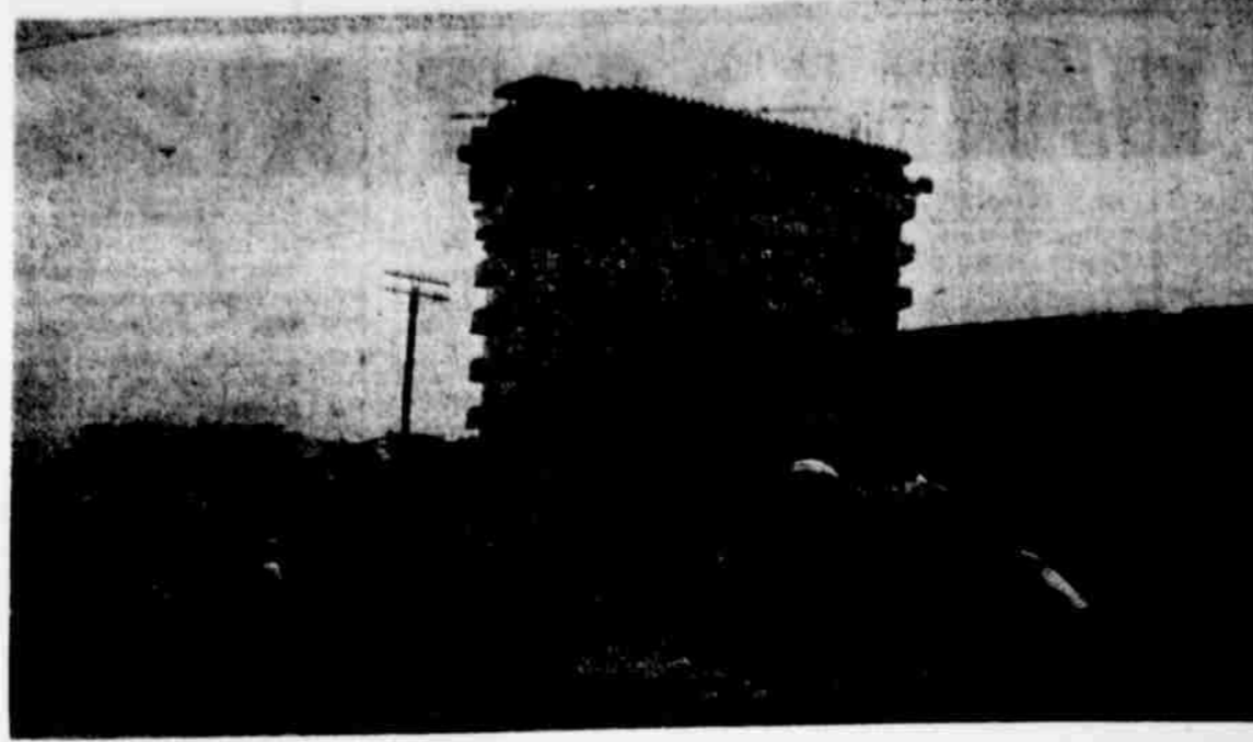
Arrival in Haskell — The Mashburn Trucking Company unloads transformer on to special equipment for the trip to the plant site.
