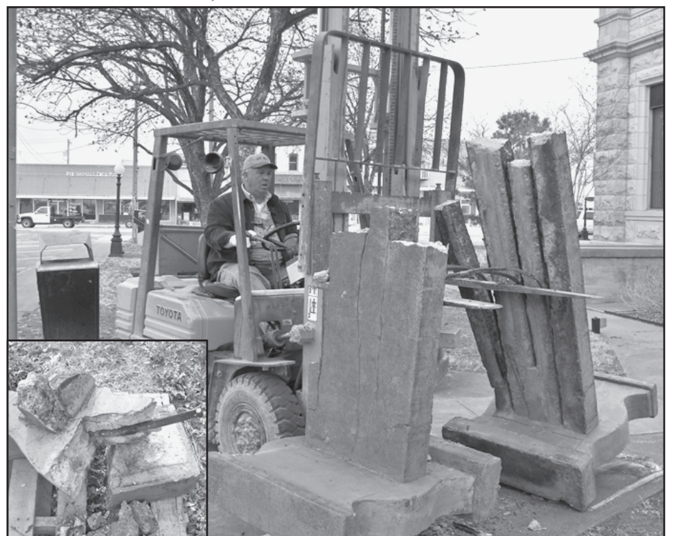
OLD BENCHES REMOVED —The old cracked benches were removed from the courthouse walks last week. County Judge David Davis lifts the bench with a forklift borrowed from Allen Moeller . New benches were installed around the courthouse square. In the inset picture, it was seen that whatever materials available were used in the construction of the old benches. This shows an automobile spring used as metal in the bench. The materials used in the supports were of varying sizes and quality. Most of the metals were rusted and deteriorated, making the benches beyond repair.
