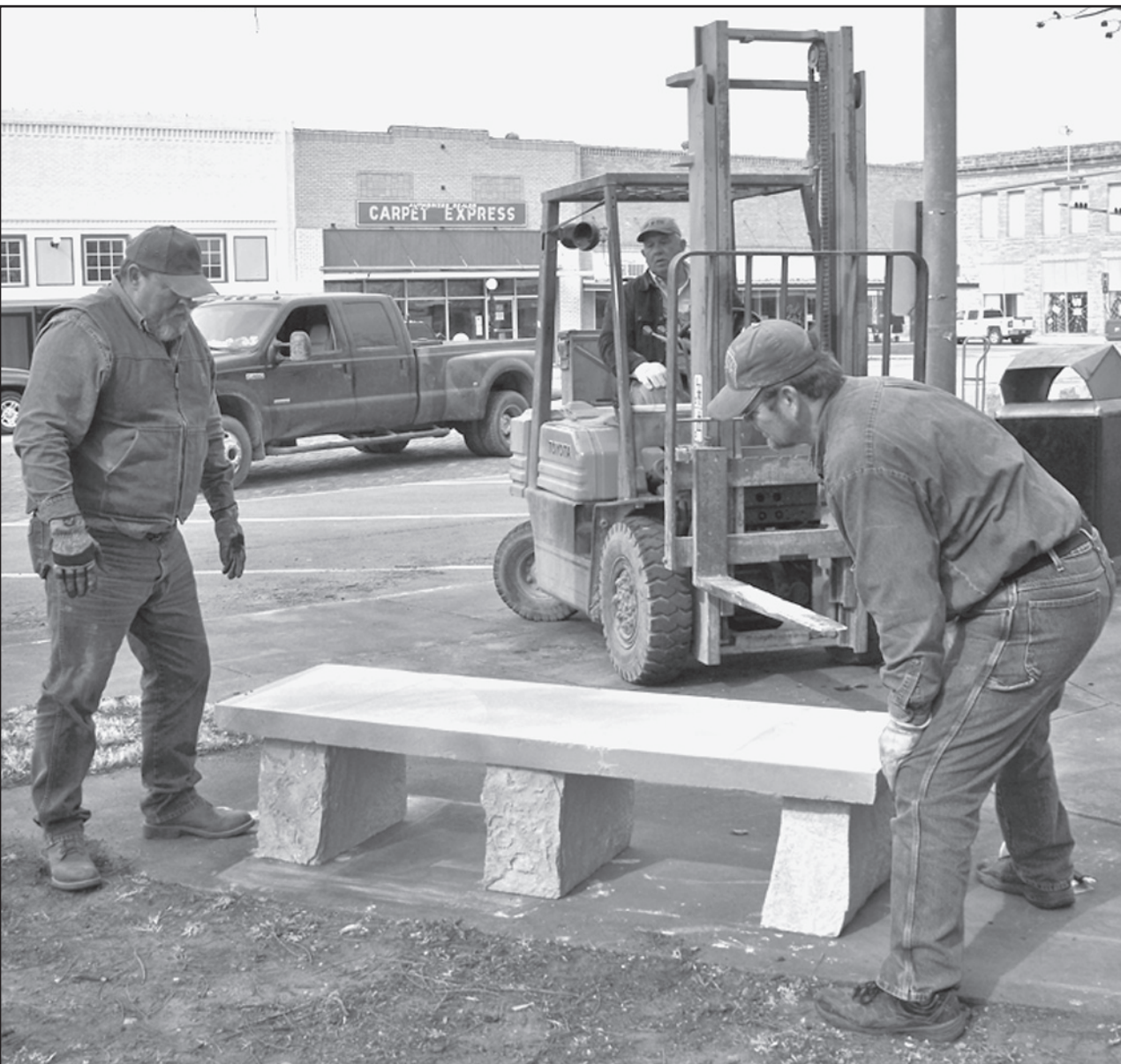
NEW BENCHES —Haskell County Commissioner Kenny Thompson, left , and county maintenance man Cameron Price, right , level the slab for the bench on rock supports after County Judge David Davis placed the slab with the forklift. The new benches were purchased from the Lueders quarry and are a beautiful complement to the stone on the courthouse building.
