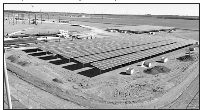
BCEC SOLAR PROJECT
