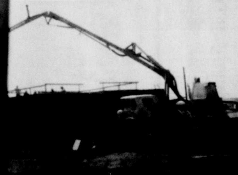
WASTE WATER TREATMENT PLANT at Millers Creek Dam is pictured as the concrete goes into the all-steel forms of the walls. (Photo courtesy of Erwin)
