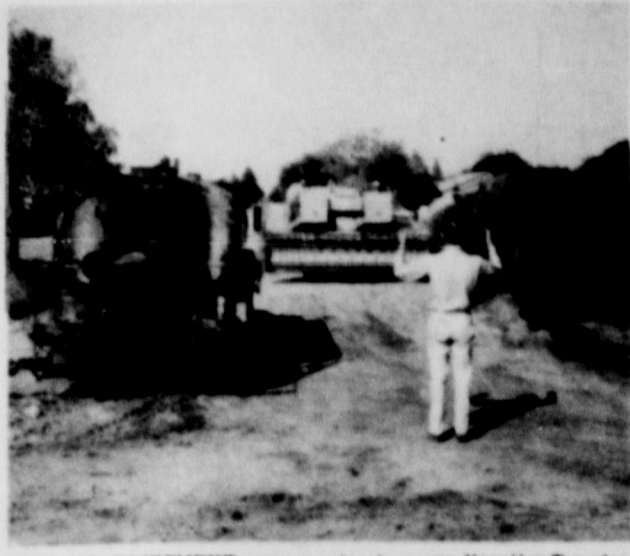
MEN AND EQUIPMENT were moving in every direction Tuesday morning as work began on the city street resurfacing. Above picture was made on South Fourth Street looking west.
