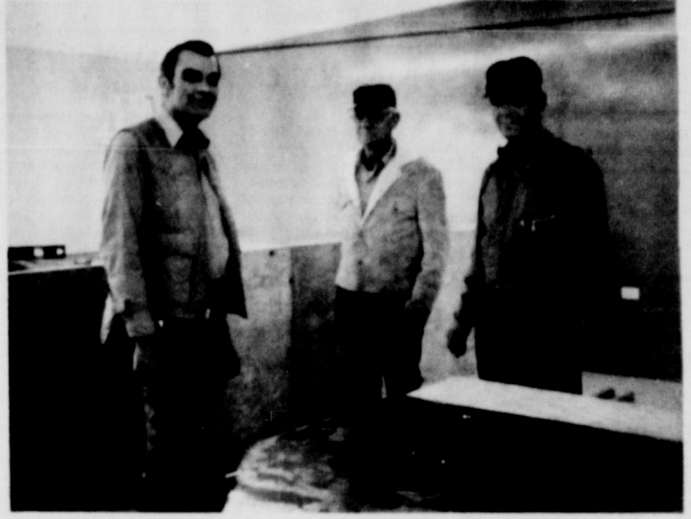
INTERRUPTING THE WORK OF THESE THREE MEN EARLY THIS WEEK, the photographer took this picture as Knox County Lumber Co. manager Jim Ross, left, observes the work of Walter Coody, center, and Carl "Dutch" Benson, both of Benjamin, as work continues on the interior of the beautiful new building.
