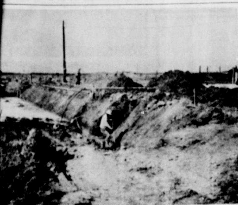
THE AERATION DITCH FOR THE WASTEWATER TREATMENT PLANT are being dug by W. B. Abbott and Co. of Lubbock. The ditch is 164 feet x 62 feet and is to be filled with a considerable amount of concrete. The city has a population of 2,000. The ditch will comply with current water quality objectives and the city must have complete treatment facilities. The project should require about three months, city officials.
