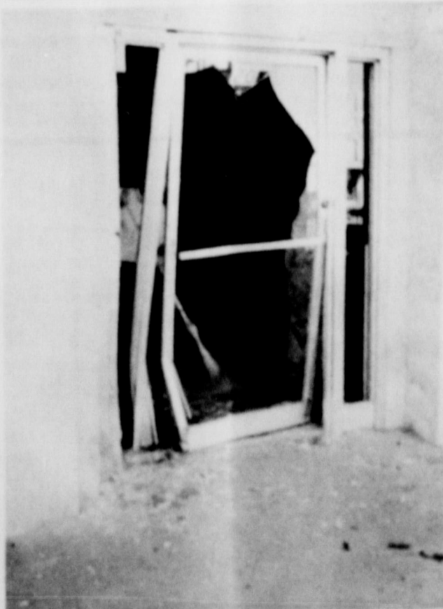
IN A CAR ACCIDENT LAST THURSDAY afternoon about 6:30 the front door of the City Hall was damaged as pictured above when a 1968 Cadillac driven by Mrs. F.E. Walker jumped the curb and hit the side of the door at an angle. Mrs. Walker said she had pulled in and jerked to remove a headscarf and her foot slipped off the brake hitting the accelerator. Mrs. Walker received a cut beneath her chin that required three stitches and the car was heavily damaged. Pictured inside the building sweeping up the broken glass are Don Railback, left, and Buddy Angle.
