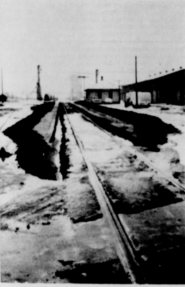
LAST FRIDAY'S SNOW was evident when the above picture was taken of the work already started in preparation of the repair to the Santa Fe railroad tracks.
