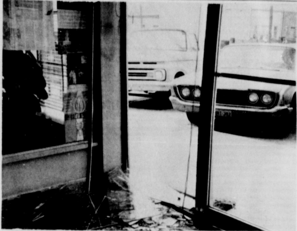
LOOKING OUT from within the U. S. Postoffice Building after the plate glass door, right in picture, and the full-length window had been demolished about two hours earlier.
