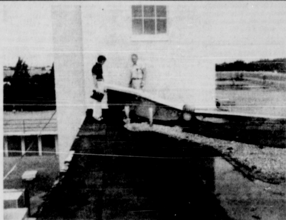
STRONG WINDS THAT HIT KNOX CITY about 10:30 Tuesday night unroofed the east wing of the second floor at the Knox County Hospital. Hospital administrator Glen Rumley, left, and custodian John Lewis stand by the metal strip that had previously trimmed the edge of the roof directly behind Rumley before the 70 to 80 mile winds ripped it loose and folded it over the roof vent at right. The damaged roof covers the hospital's operating room, delivery room and nursery. Rain in Knox City during the thunderstorm measured .40.
