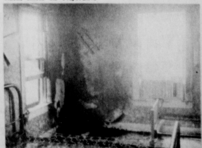
WHERE THE FIRE STARTED — Shown above is the back bedroom of the Wesley Robbins' residence which was heavily damaged by fire Wednesday afternoon of last week.
