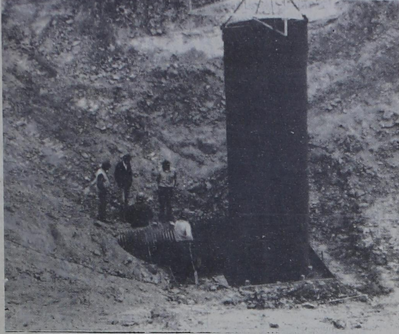
GRADE STABILIZATION STRUCTURE on the farm of W. R. Moore, Jr., has protected the farmland from a gully that was eating into the land. Moore accomplished this work by entering in the Great Plains Program with the Soil Conservation Service. He has also built parallel terraces, diversion terraces, waterways, and put in underground irrigation pipe. The farm receiving the improvements is located southwest of Knox City.
