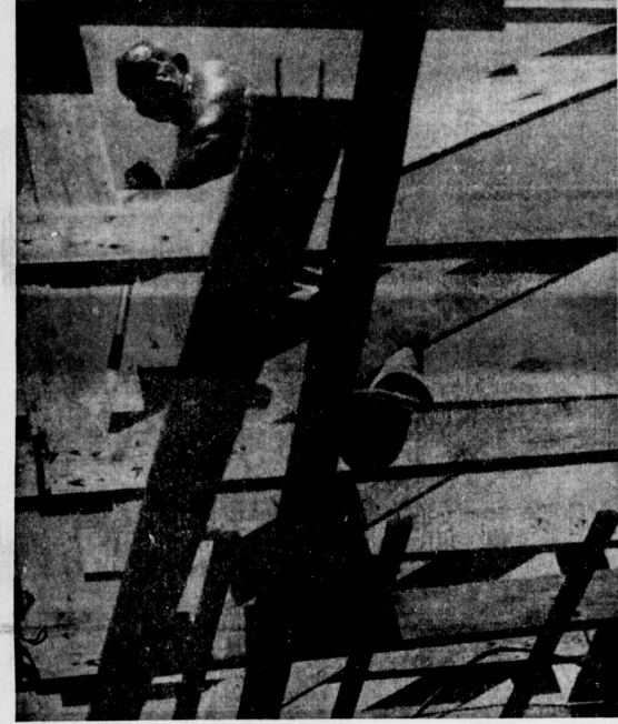
OLD DESHAZO BITES THE DUST — It's curtains for one of Muleshoe's earliest school buildings. West Deshazo Roof-already is gone and workmen have started tearing out the rafters. This is Hank Weber, Muleshoe, as he tackles one of the 20's with a wrecking bar. (Journal Photo)
