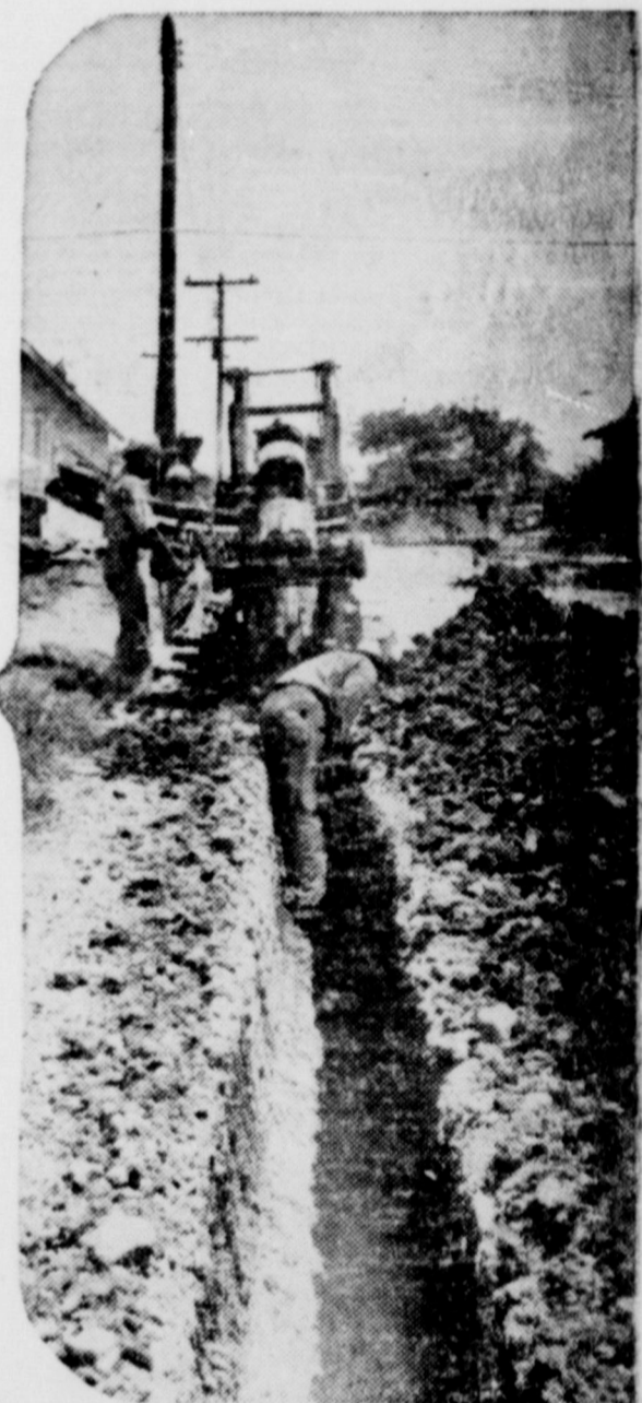
Ditching machine is major unit of highly mechanized teams who build new distribution lines in towns and cities on Lone Star Gas System.
